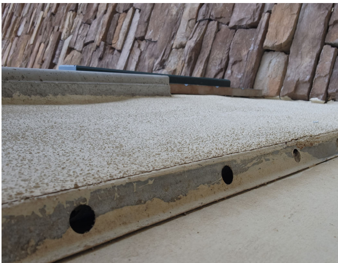
However, ventilation holes in the weep screed may allow flames into the walls of a structure.
